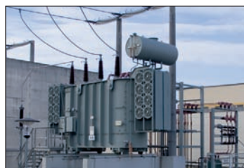
real image of a transformer
